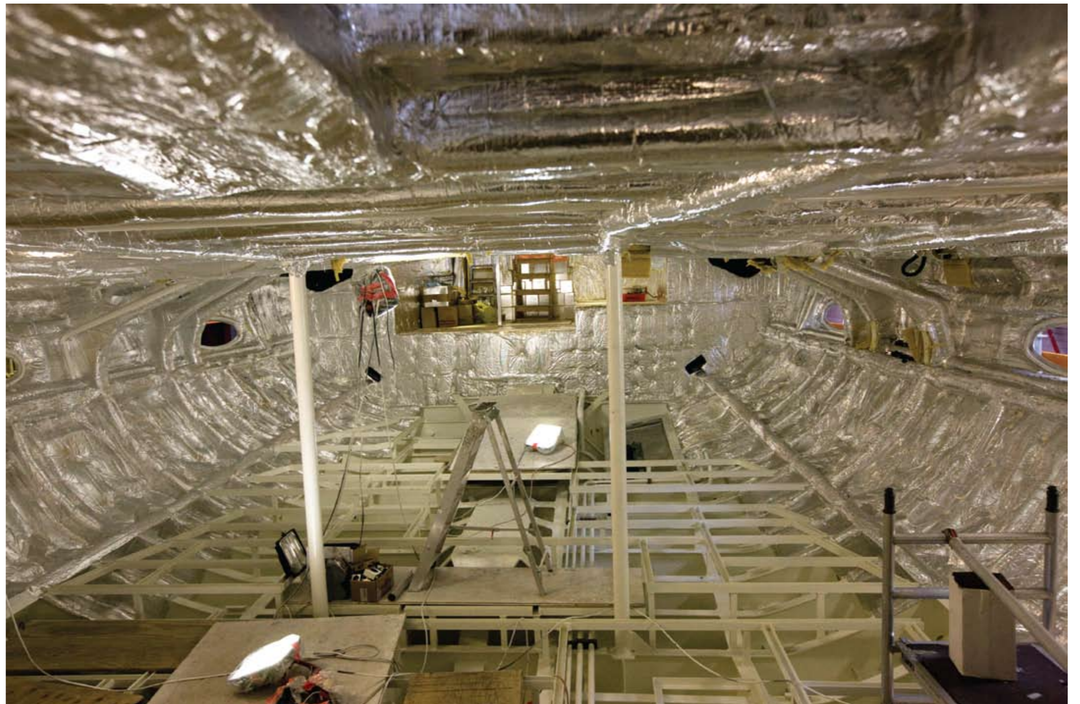
ABOVE The vast carcass of the 172ft/52m ketch Marie . The silver lining insulates the aluminium hull. This shot was taken in 2009. Launch date is spring 2010.
